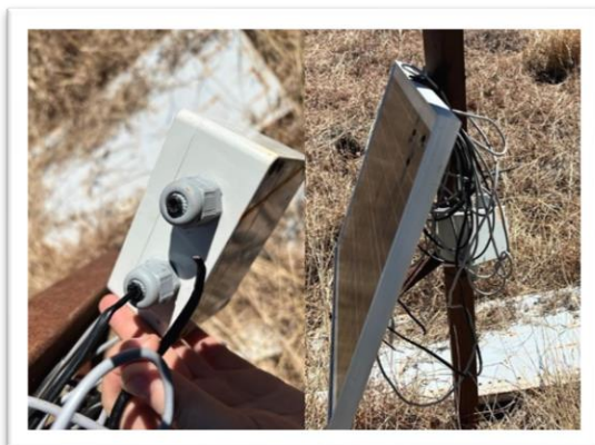
Figure 56 - Cable Damage from Native Bush Rats to Noise Monitor Solar Panel.
