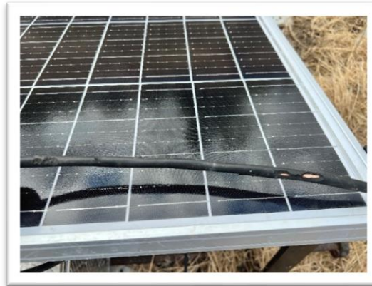
Figure 55 - Cable Damage from Native Bush Rats to Weather Station Solar Panel.
