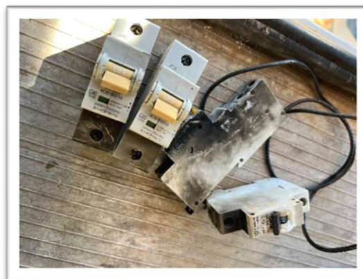
Figure 9 - Rat Damage to Saint Elmo Homestead Power Supply (July 2024).
